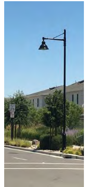
Collector/Residential Street Lights
